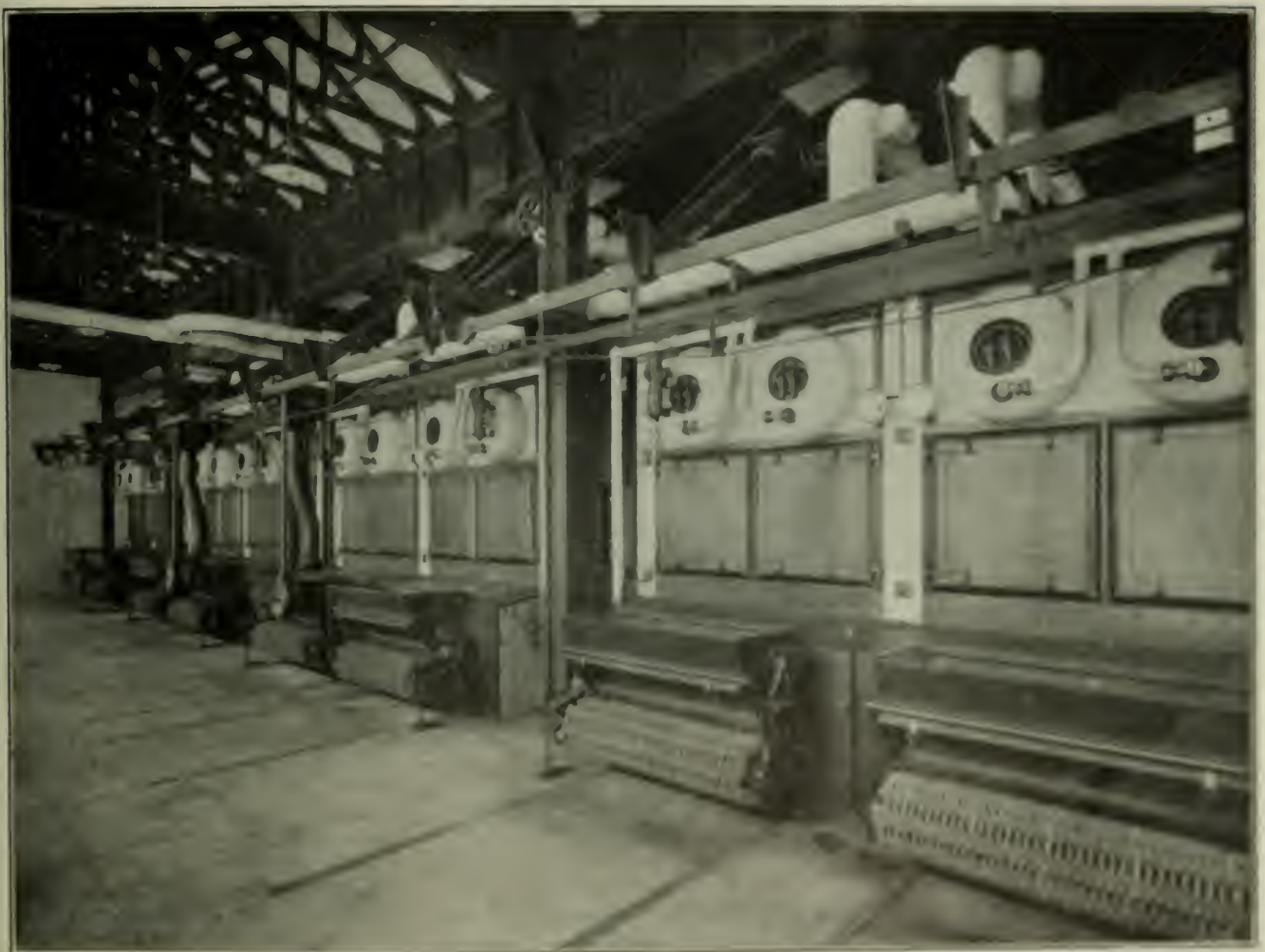
FIG. 1. THE BOILER INSTALLATION
